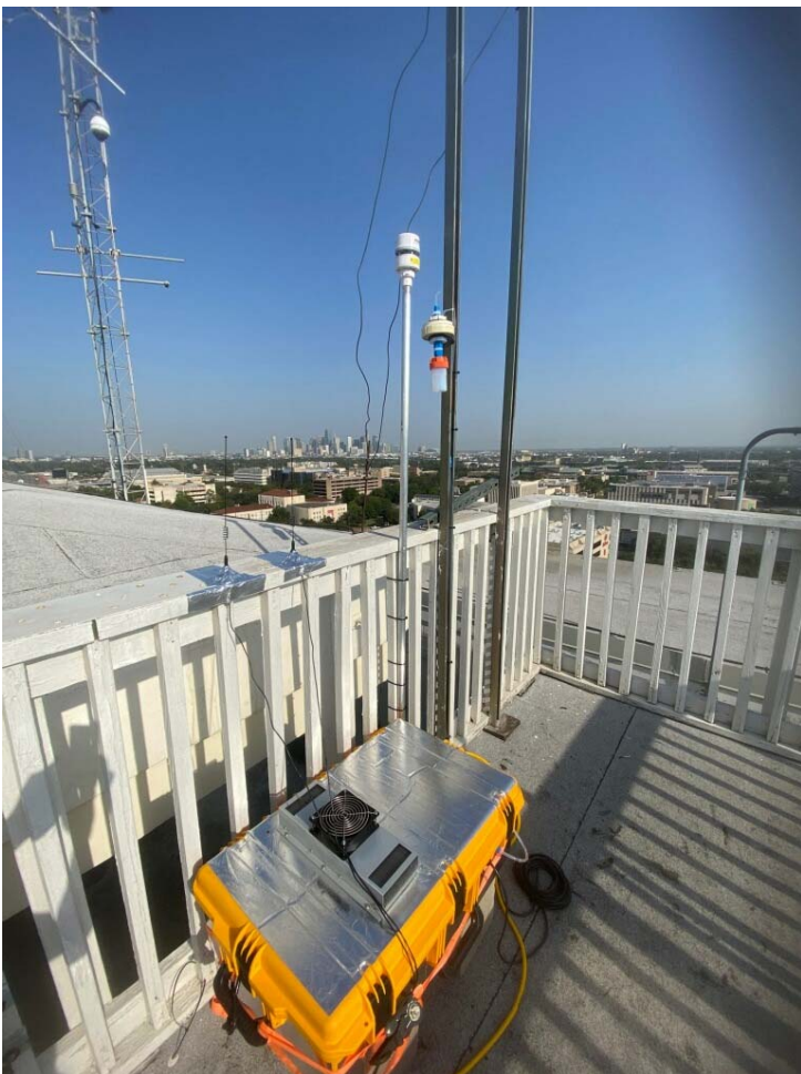
Figure 20-0042. GO3 sample box on the roof of a Moody Tower lab trailer with met sensor and inlet. The main Moody Tower (C695) sample mast is in the background where O 3 and met parameters are measured for C695.
